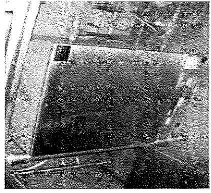
Electric hot water booster heater
