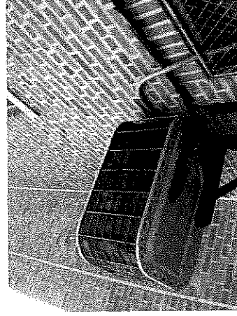
Briarcliff MS Heat Pump AC Unit
