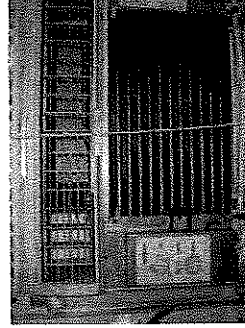
Lake Drive School: Typical Window AC Unit
